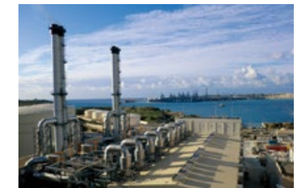
Diesel Engine Generating Plant
